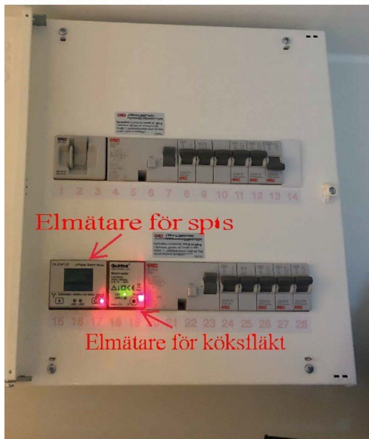
Switchboard, electricity meter for the kitchen stove and the kitchen fan
