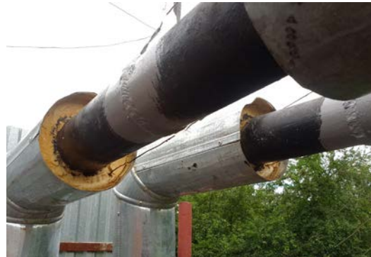
Photo: new isolated pipes Source Shorthand social)
