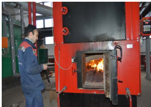
Photo: Kriger boiler, 3*820 KWt Source Zhovkvateploenergo
