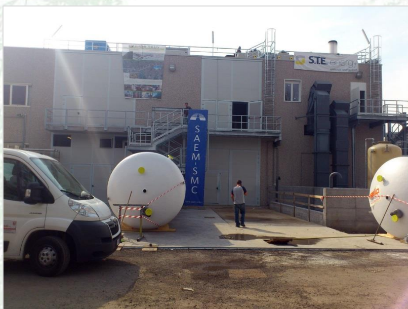
Figure 45 - Prometeo biomass CHP plant on the outskirts of Milan
