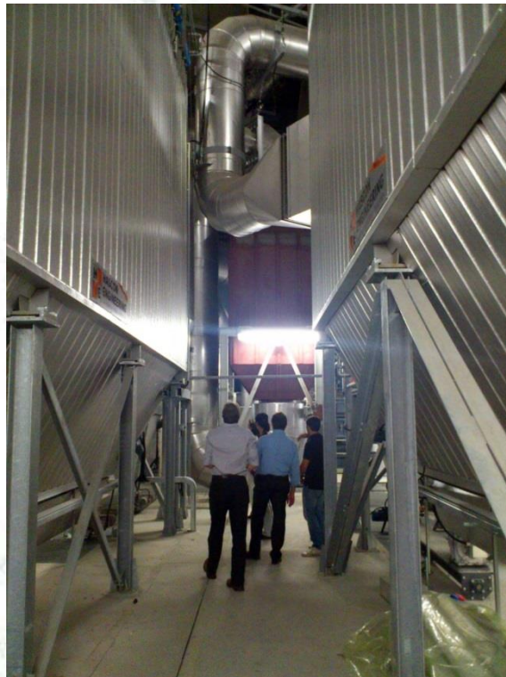
Figure 21 - Prometheus project, between the air filtration units
