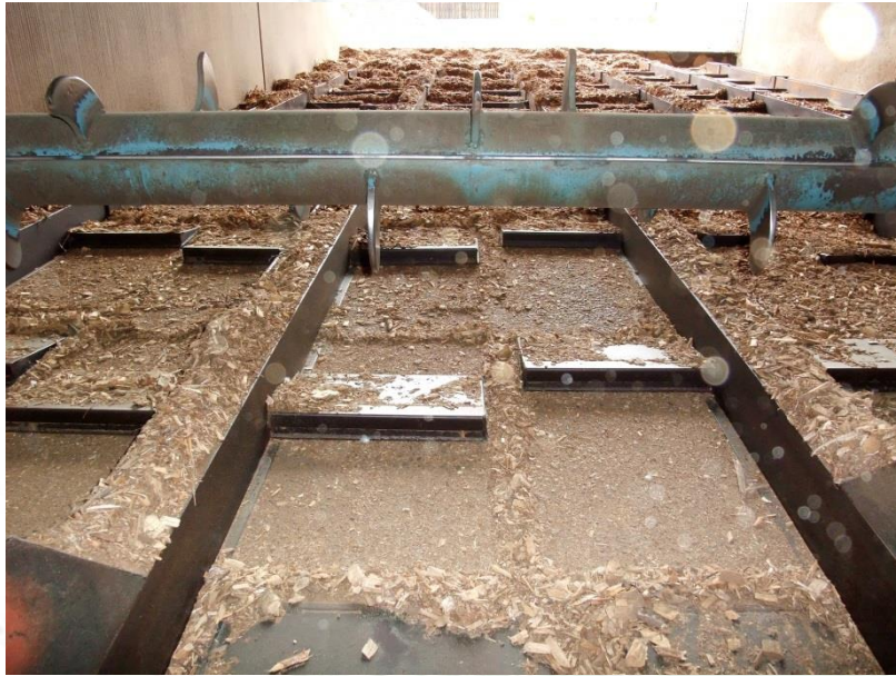
Figure 26 - Walking floor at Braås district heating plant; in cold weather chip are frozen solid and need to be broken up
