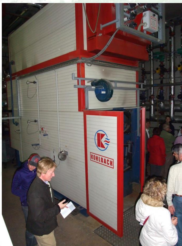
Figure 24 – 1.2 MW biomass boiler sited in a bunker at the Fröhling factory
