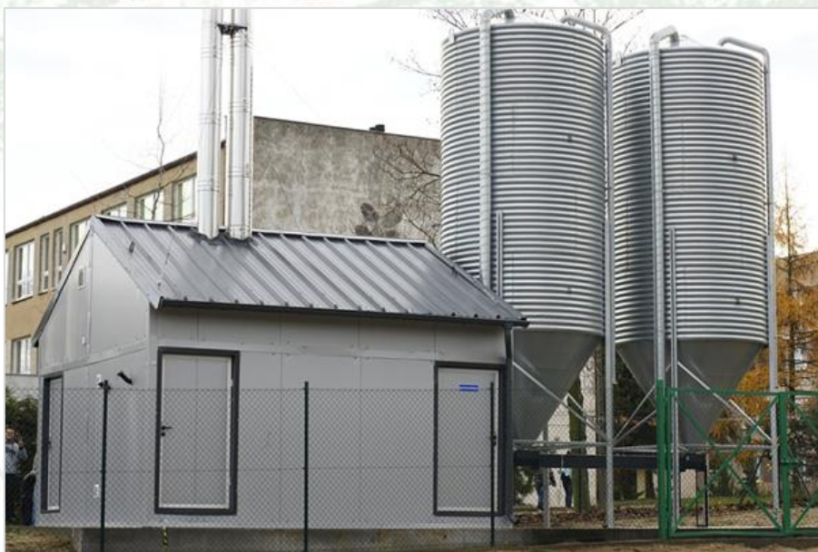
Figure 33 - Containerised pellet-fired boiler house in Owidz
