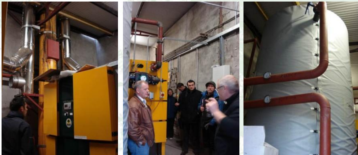
Figure 49 - Gurteen Agricultural College, biomass boilers and thermal accumulator tank
