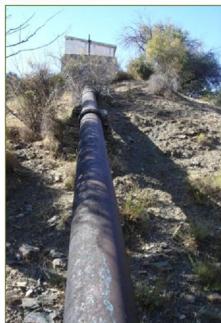
Figure 47: Penstock, Central Alhori I. Granada
