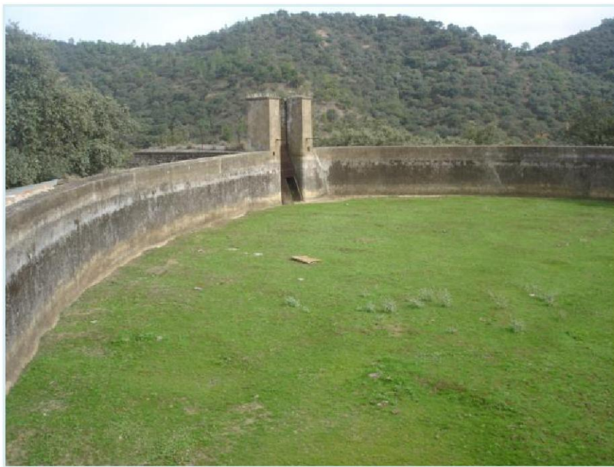
Picture 12. Forebay. Santa Teresa Small-hydropower plant. La Nava Huelva
