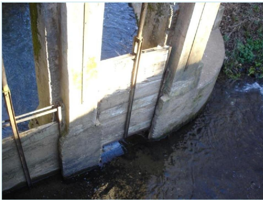
Picture 15. Gates. Santa Teresa small-hydropower plant. La Nava. Huelva
